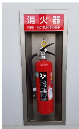
powder fire extinguisher
